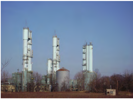
Praxair towers (existing)
